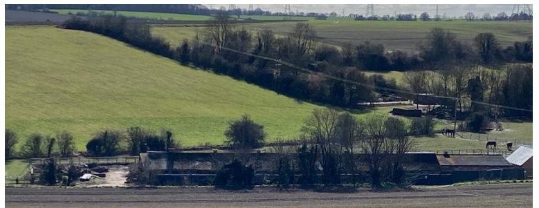
11 th March 2023 the start of the demolition of the Old Piggeries, the large Willow tree has been felled and site starting to be cleared
